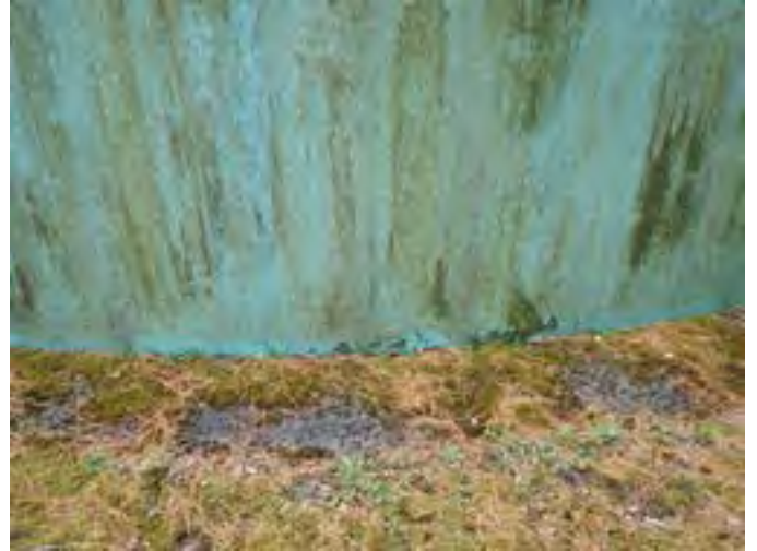
16 Foundation Found Below Grade And Covered With Moss And Vegetation
