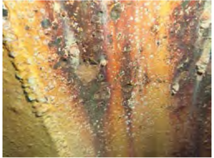
68 Wall Panel Having Pitting Of The Steel
