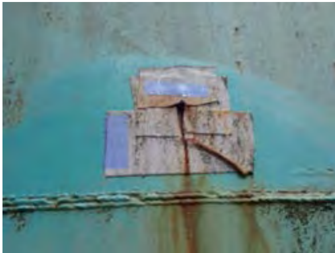
3 Wood Dowel And Patch Temporarily Sealing A Penetration In The Second Wall Panel On The Southernmost Side Of The Tank
