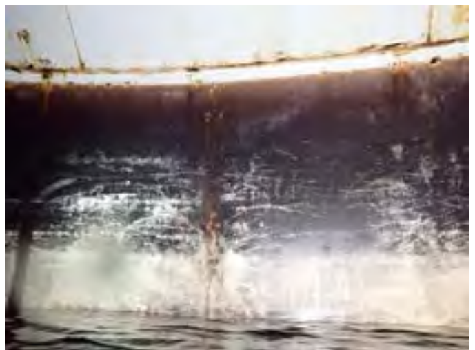
60 Interior Wall Having Exposed Steel And Corrosion
