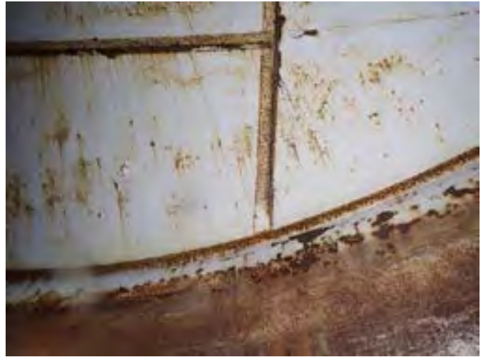
80 Interior Wall Having Coating Loss, Exposed Steel And Corrosion
