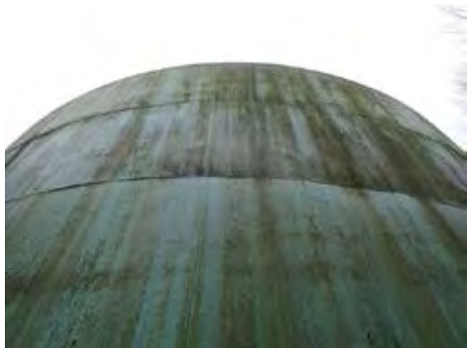
12 Exterior Wall Having Coating Loss, Exposed Steel, Corrosion And Accumulated Mildew
