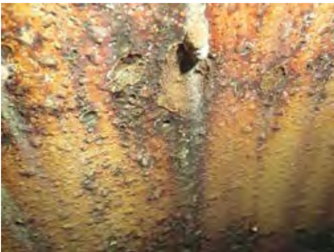
71 Wall Panel Having Pitting Of The Steel
