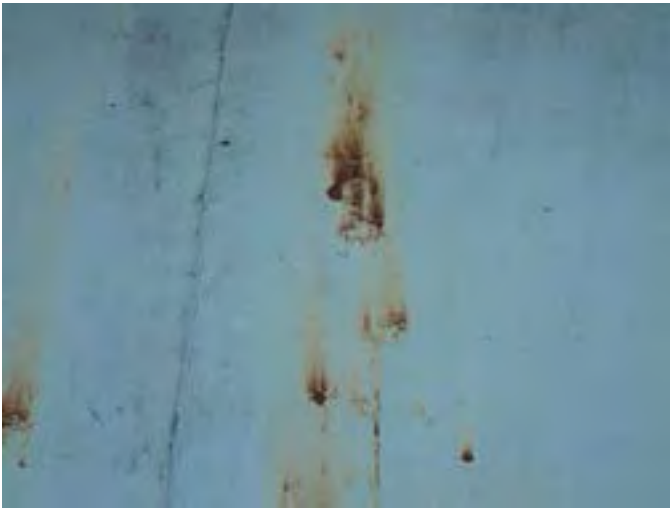
33 Roof Having Coating Loss, Exposed Steel, Corrosion And A Non-Uniform Accumulation Of Mildew
