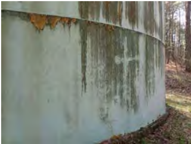
3 Exterior Wall Having Coating Loss, Exposed Primary Coating And Accumulated Mildew
