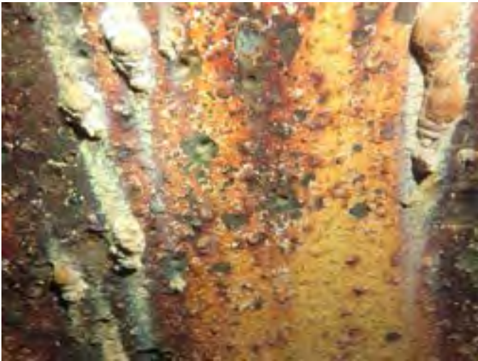
69 Wall Panel Having Pitting Of The Steel
