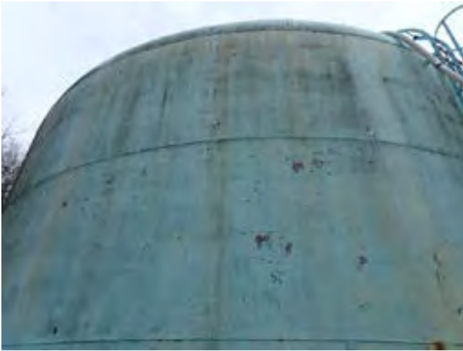
7 Exterior Wall Having Coating Fatigue, Exposed Primary Coating, Exposed Steel And Corrosion
