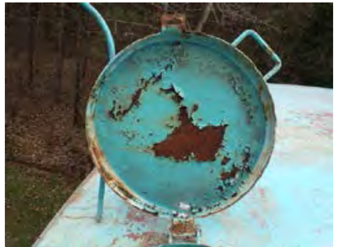
36 Interior Of The Hatch Cover Having Exposed Steel And Corrosion
