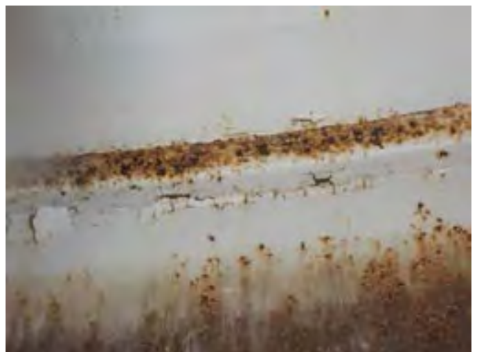
78 Interior Wall Having Coating Loss, Exposed Steel And Corrosion
