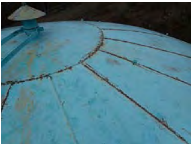
23 Roof Having Exposed Primary Coating, Exposed Steel And Corrosion
