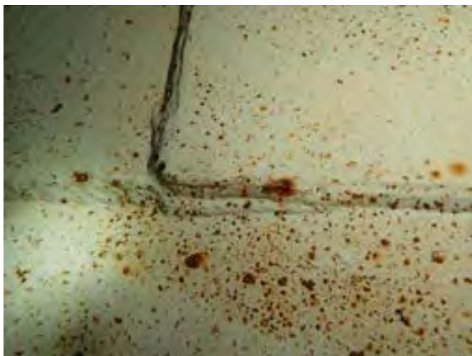
47 Floor Having Coating Loss, Exposed Steel And Corrosion
