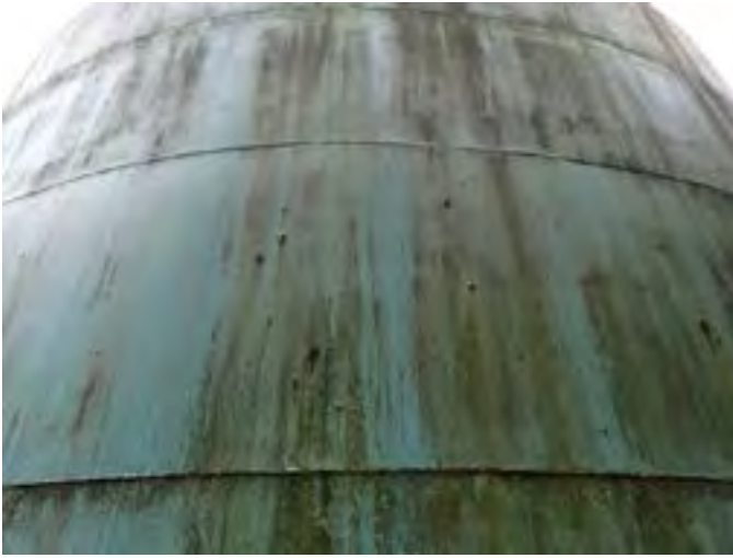
13 Exterior Wall Having Coating Loss, Exposed Steel, Corrosion And Accumulated Mildew
