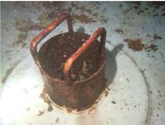
51 Removable Slit Stop Riser Having Exposed Steel And Corrosion
