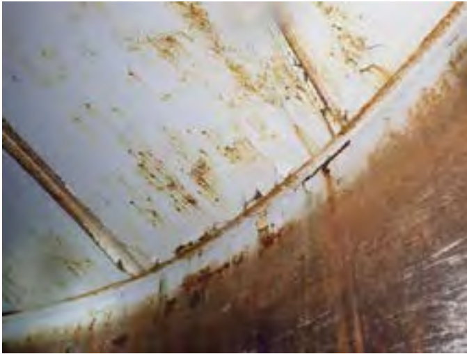
79 Interior Wall Having Coating Loss, Exposed Steel And Corrosion
