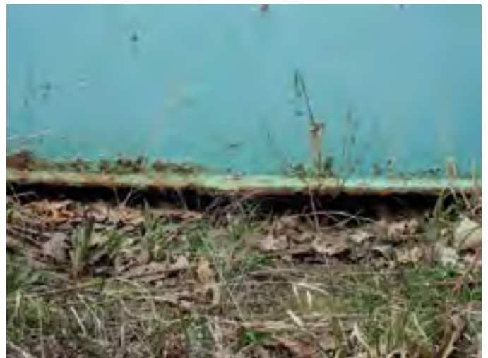
12 Exterior Wall Having Coating Fatigue, Exposed Primary Coating, Exposed Steel And Corrosion
