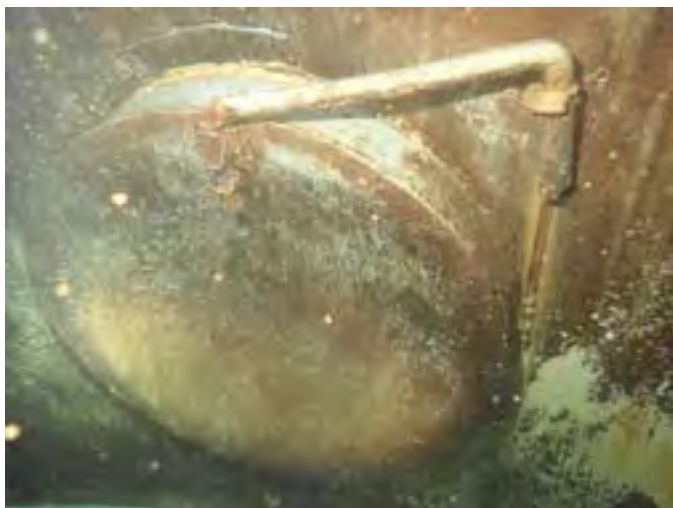
47 Manway Having Coating Loss, Exposed Steel And Corrosion
