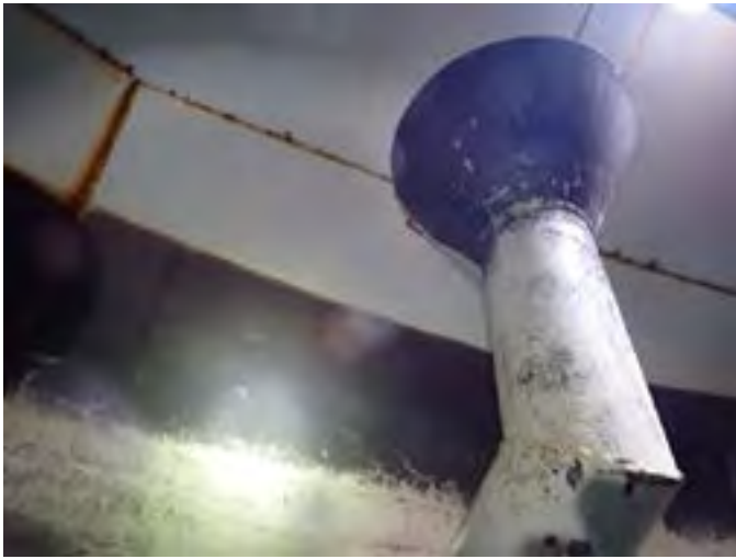
73 Overflow Pipe Having Exposed Steel And Corrosion
