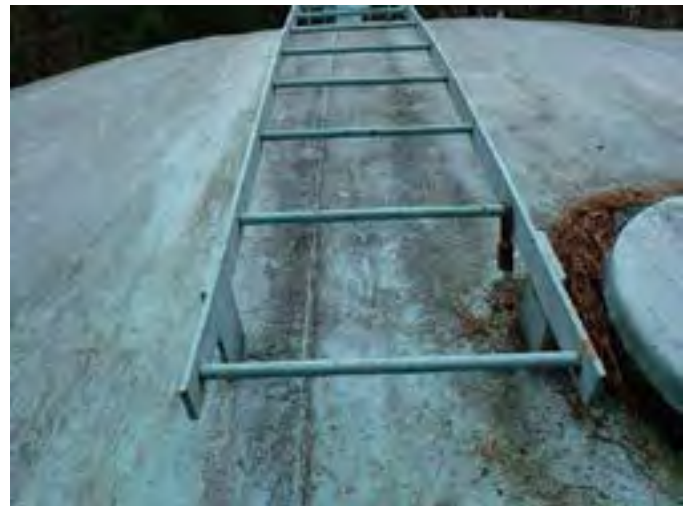
24 Vent Access Ladder Having Exposed Steel And Corrosion
