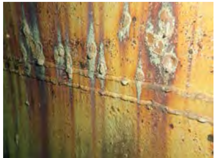
66 Interior Wall Having Coating Loss, Exposed Steel And Corrosion
