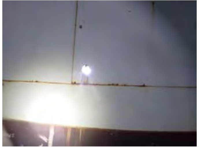
68 Overhead Having Exposed Steel, Corrosion And An Open Rigging Hole Penetration
