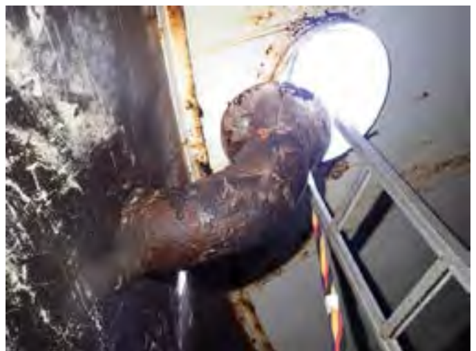
72 Overflow Pipe Having Exposed Steel And Corrosion
