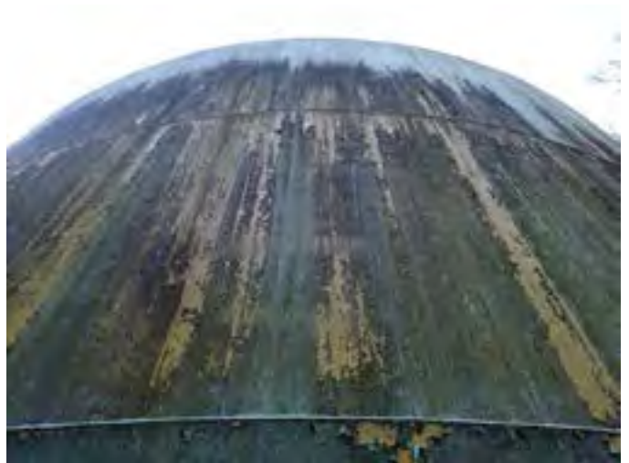
6 Exterior Wall Having Coating Loss, Exposed Primary Coating And Accumulated Mildew
