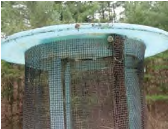
35 Vent Assembly Having Exposed Steel And Corrosion
