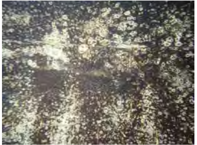
56 Interior Wall Having Exposed Steel And Corrosion
