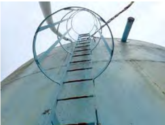
17 Ladder And Safety Cage Having Exposed Primary Coating, Exposed Steel And Corrosion
