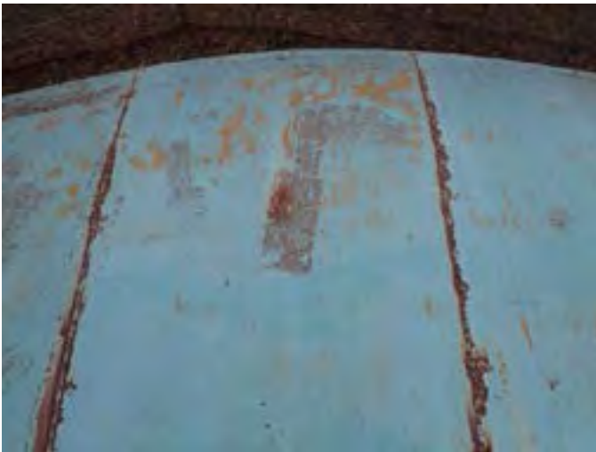
27 Roof Having Exposed Primary Coating, Exposed Steel And Corrosion
