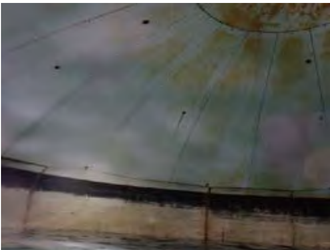
71 Overhead Having Surface Corrosion And Exposed Steel
