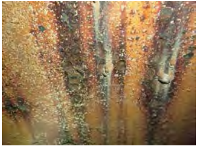
74 Wall Panel Having Pitting Of The Steel
