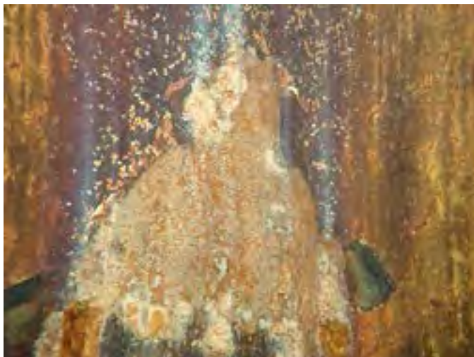
65 Interior Wall Having Coating Loss, Exposed Steel And Corrosion
