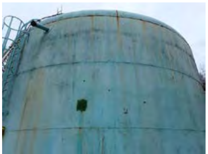
4 Steel Patch Welded To A Wall Panel Having Minimal Leakage
