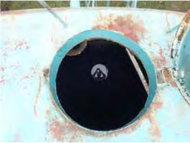
37 Interior Of The Hatch Trunk Having Exposed Steel And Corrosion
