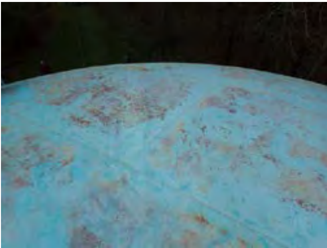
27 Roof Having Coating Fatigue, Exposed Primary Coating, Exposed Steel And Corrosion
