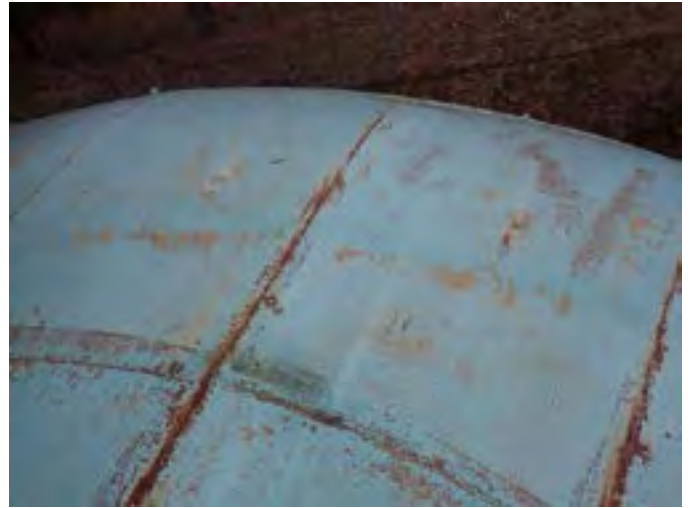
26 Roof Having Exposed Primary Coating, Exposed Steel And Corrosion
