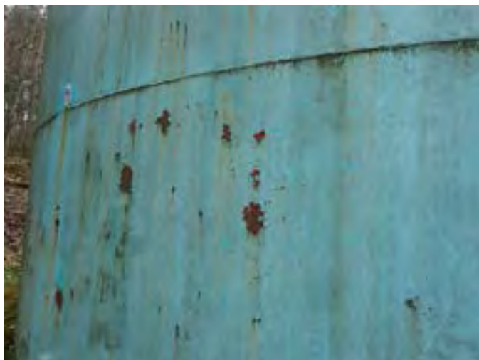
5 Exterior Wall Having Coating Loss, Exposed Primary Coating, Exposed Steel, Corrosion And Accumulated Mildew
