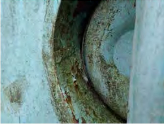
19 Manway Having Exposed Steel And Corrosion
