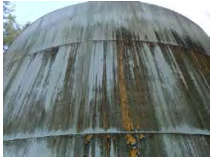
10 Exterior Wall Having Coating Loss, Exposed Primary Coating And Accumulated Mildew
