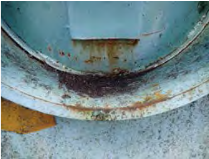
21 Manway Having Exposed Steel And Corrosion
