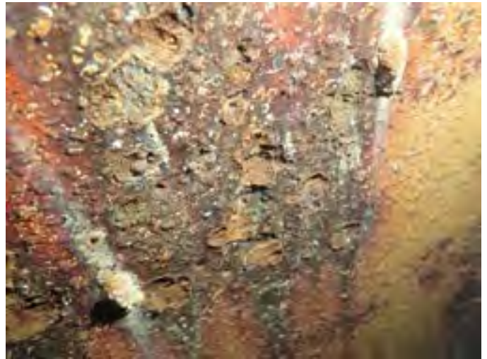
70 Wall Panel Having Pitting Of The Steel
