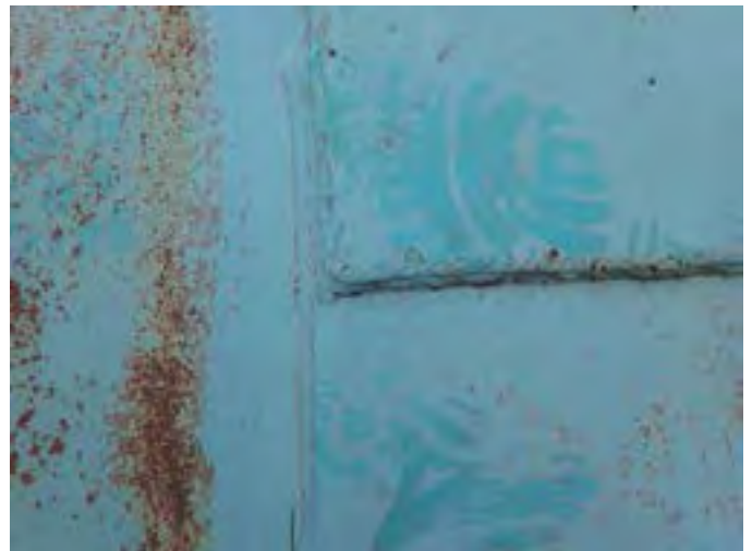
30 Roof Having Coating Fatigue, Exposed Primary Coating, Exposed Steel And Corrosion
