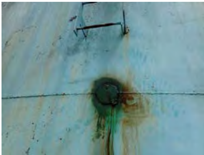
3 Steel Patch Welded Over A Weld Found Without Leakage
