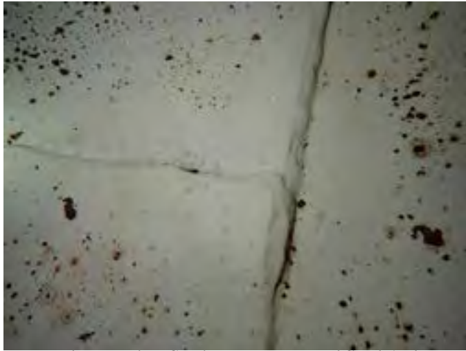
45 Floor Having Coating Loss, Exposed Steel And Corrosion
