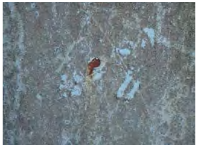
12 Exterior Wall Having Coating Loss, Exposed Steel And Corrosion
