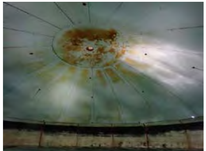
66 Overhead Having Surface Corrosion Showing Through The Coating
