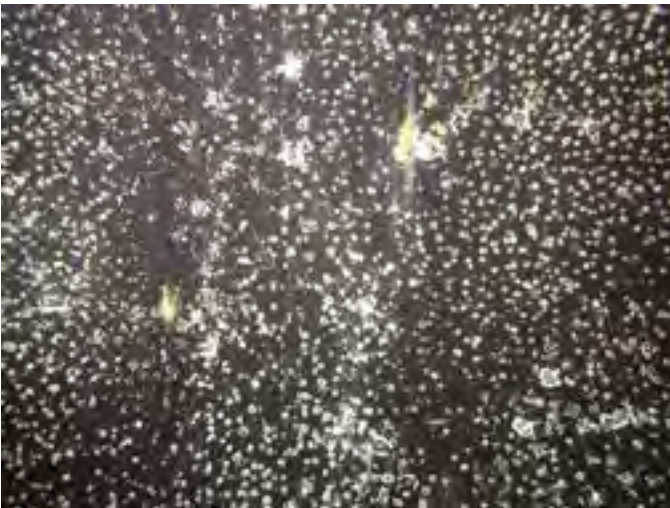
51 Interior Wall Having Exposed Steel And Corrosion
