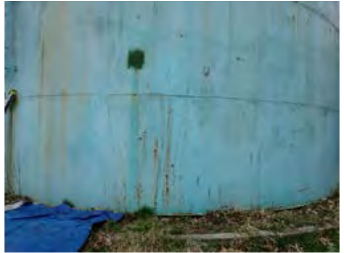
8 Exterior Wall Having Coating Fatigue, Exposed Primary Coating, Exposed Steel And Corrosion
