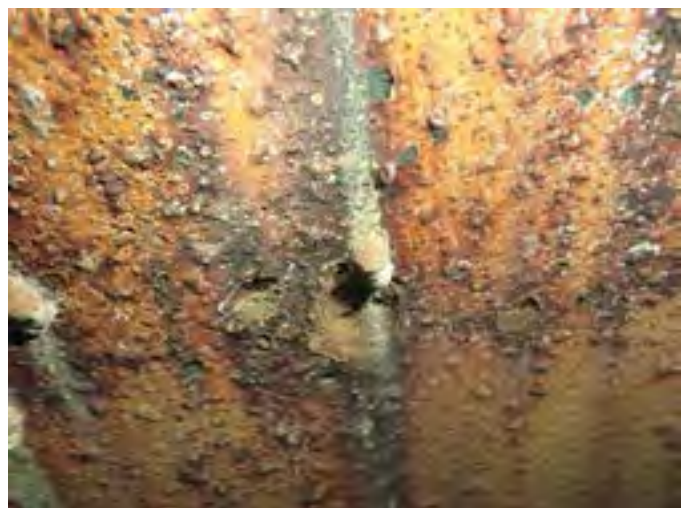
72 Wall Panel Having Pitting Of The Steel
