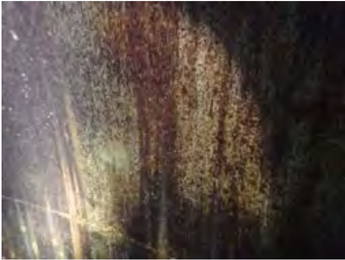
61 Interior Wall Having Coating Fatigue, Exposed Steel And Corrosion
