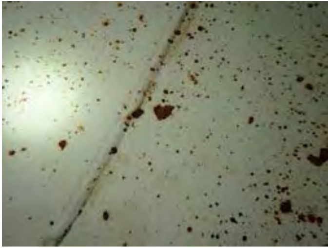
43 Floor Having Coating Loss, Exposed Steel And Corrosion
