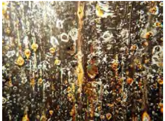
64 Third Row Of Wall Panels Above The Tank Floor Having Pitting Of The Steel
