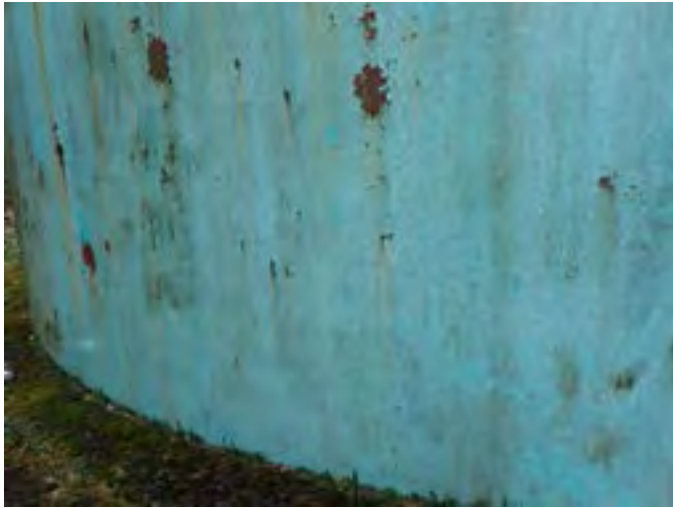
7 Exterior Wall Having Coating Loss, Exposed Primary Coating, Exposed Steel, Corrosion And Accumulated Mildew
