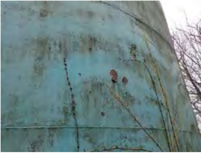
13 Exterior Wall Having Coating Fatigue, Exposed Primary Coating, Exposed Steel And Corrosion
