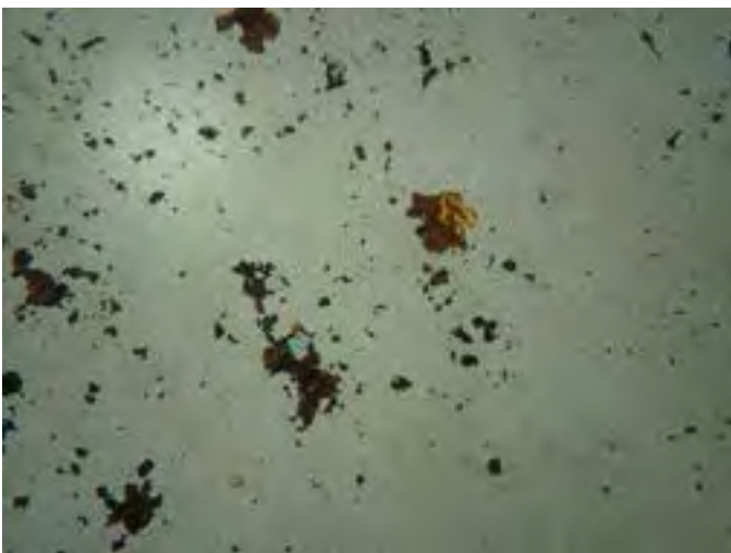
41 Floor Having Coating Loss, Exposed Steel And Corrosion
