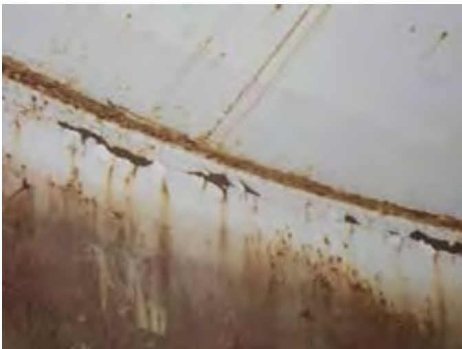
77 Interior Wall Having Coating Loss, Exposed Steel And Corrosion
