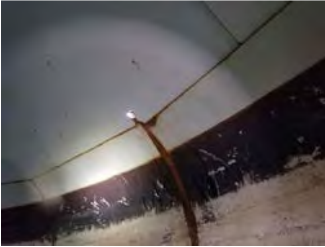
67 Overhead Having Exposed Steel, Corrosion And An Open Rigging Hole Penetration
