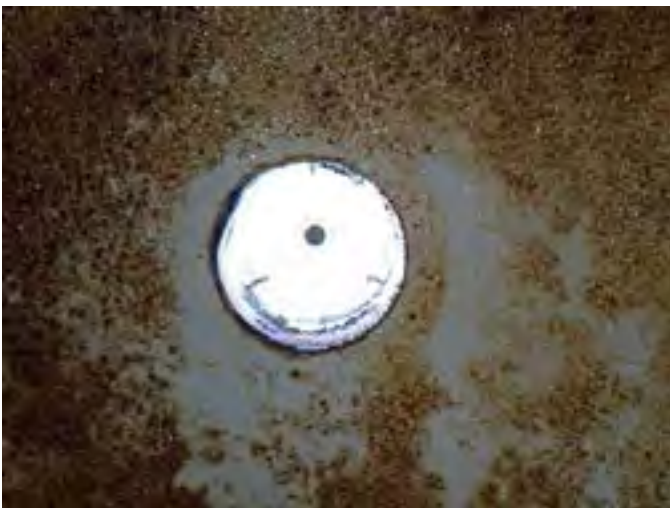
71 Overhead Having Coating Loss, Exposed Steel And Corrosion
