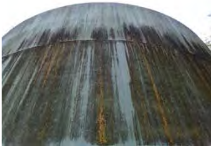
9 Exterior Wall Having Coating Loss, Exposed Primary Coating And Accumulated Mildew
