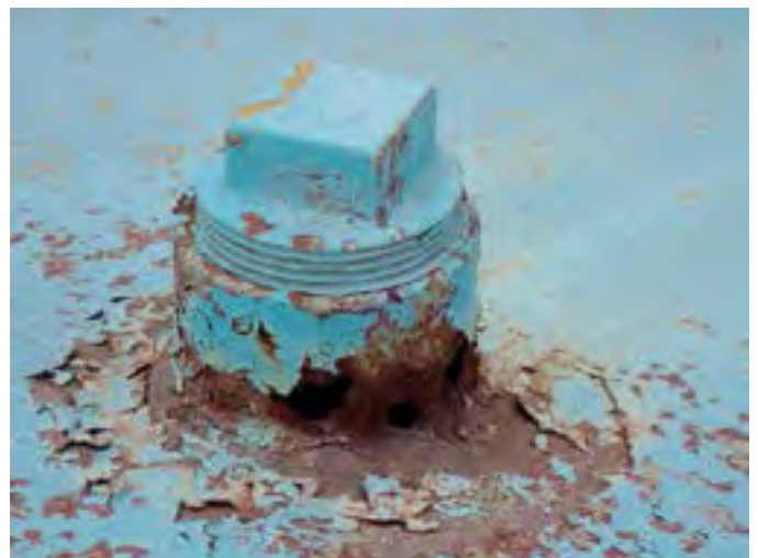
30 Deteriorating Rigging Hole Coupling
