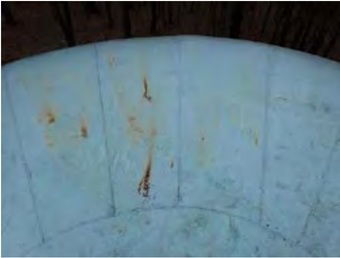
31 Roof Having Coating Loss, Exposed Steel, Corrosion And A Non-Uniform Accumulation Of Mildew
