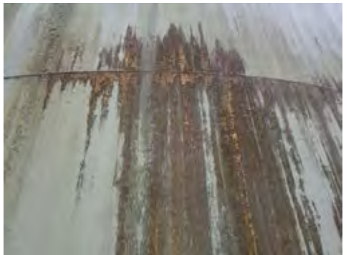
4 Exterior Wall Having Coating Loss, Exposed Primary Coating And Accumulated Mildew
