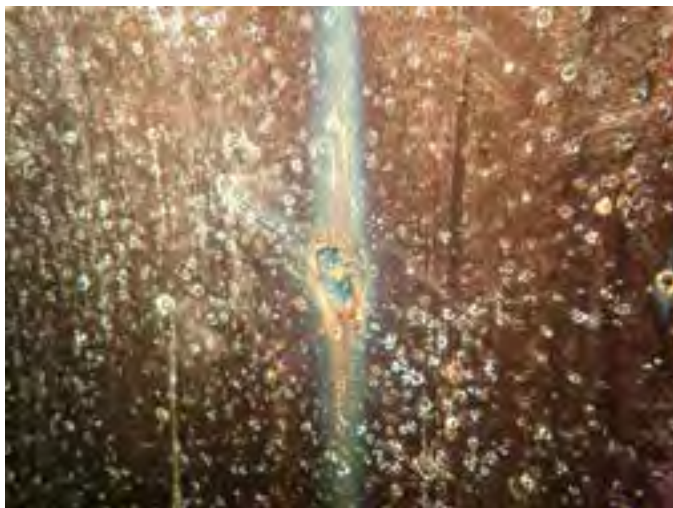
65 Interior Wall Having Pitting Of The Steel
