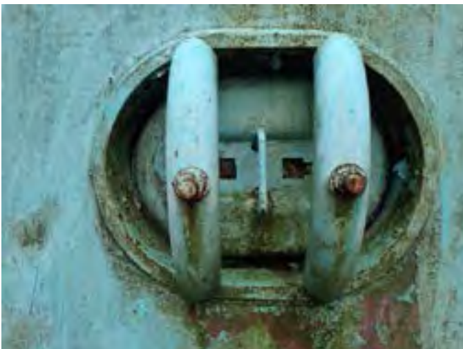
17 Manway Having Coating Fatigue
