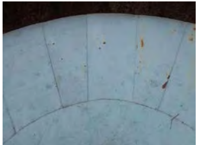
30 Roof Having Coating Loss, Exposed Steel, Corrosion And A Non-Uniform Accumulation Of Mildew
