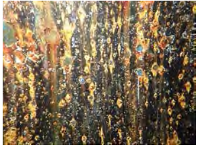
62 Third Row Of Wall Panels Above The Tank Floor Having Pitting Of The Steel
