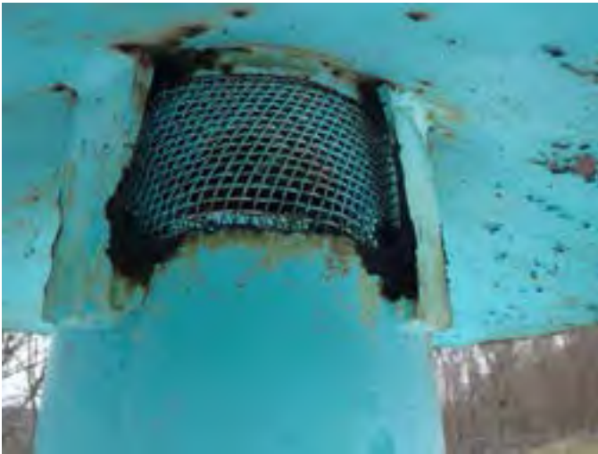
33 Vent Assembly Having Exposed Primary Coating, Exposed Steel And Corrosion
