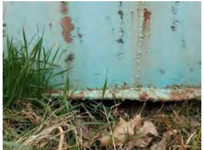
10 Exterior Wall Having Coating Fatigue, Exposed Primary Coating, Exposed Steel And Corrosion
