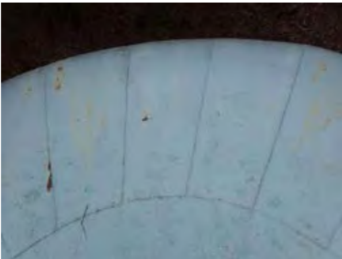
29 Roof Having Coating Loss, Exposed Steel, Corrosion And A Non-Uniform Accumulation Of Mildew
