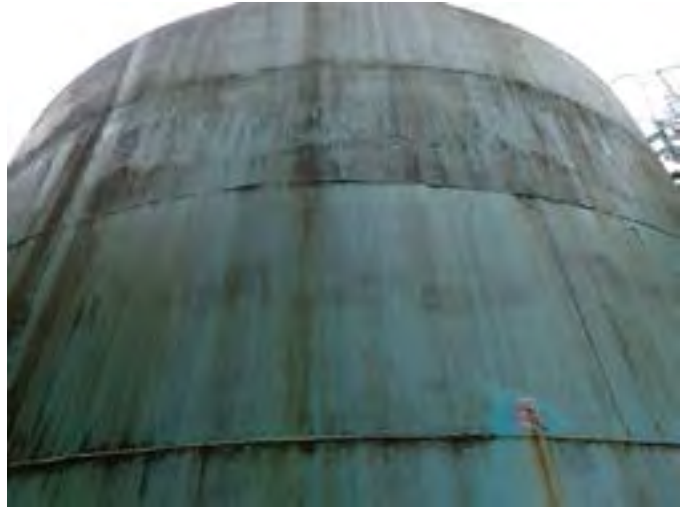
8 Exterior Wall Having Coating Loss, Exposed Primary Coating, Exposed Steel, Corrosion And Accumulated Mildew
