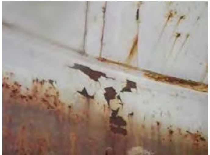
76 Interior Wall Having Coating Loss, Exposed Steel And Corrosion
