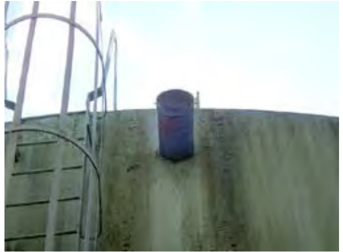
26 Overflow Pipe Having Exposed Primary Coating, Exposed Steel And Corrosion
