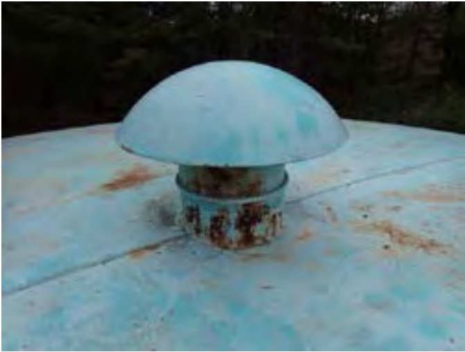
31 Vent Assembly Having Coating Loss, Exposed Steel And Corrosion
