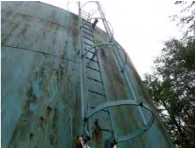
21 Ladder And Safety Cage Having Coating Loss, Exposed Steel And Corrosion
