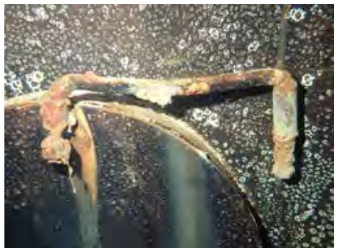
48 Manway Having Exposed Steel And Corrosion
