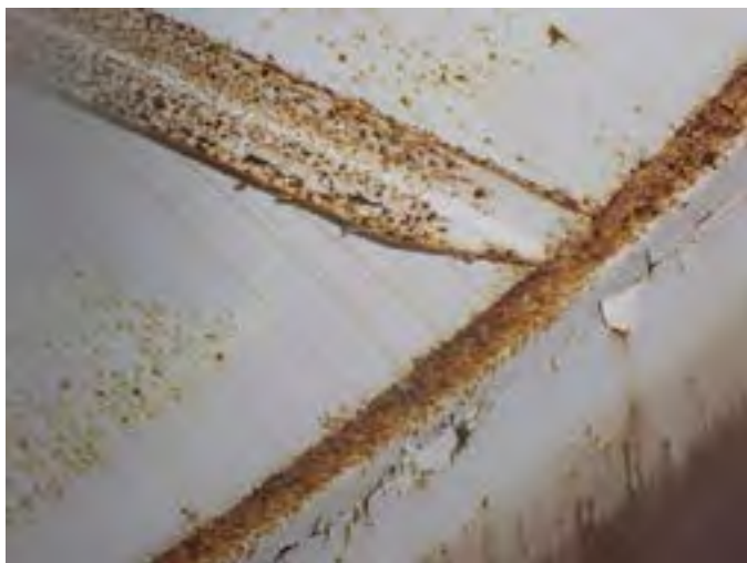
83 Overhead Having Coating Loss, Exposed Steel And Corrosion
