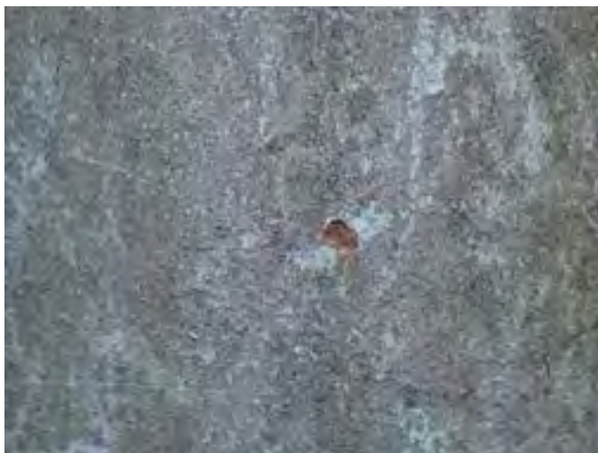
11 Exterior Wall Having Coating Loss, Exposed Steel And Corrosion
