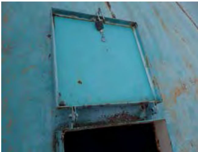
35 Interior Of The Hatch Cover Having Exposed Steel And Corrosion
