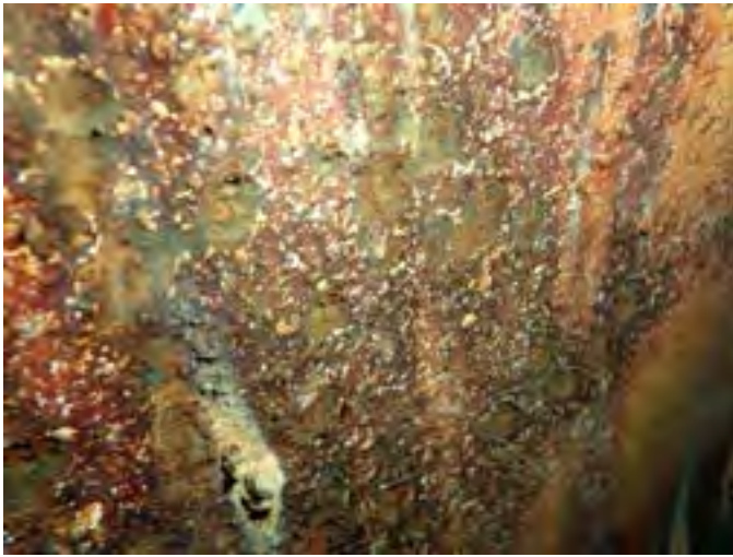
73 Wall Panel Having Pitting Of The Steel
