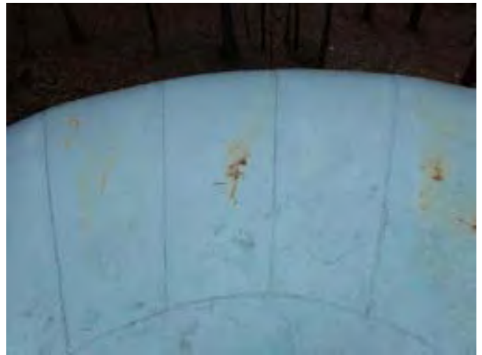
28 Roof Having Coating Loss, Exposed Steel, Corrosion And A Non-Uniform Accumulation Of Mildew
