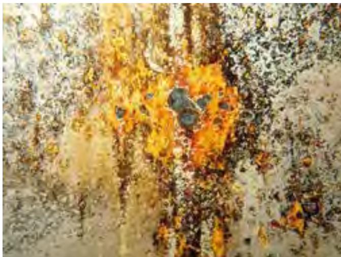
65 Third Row Of Wall Panels Above The Tank Floor Having Pitting Of The Steel
