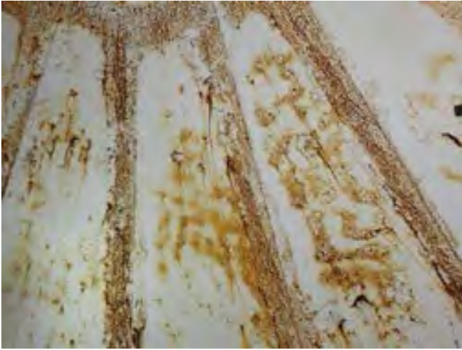
67 Overhead Having Coating Loss, Exposed Steel And Corrosion
