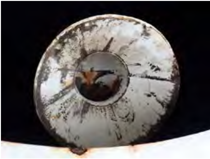
73 Unobstructed Overflow Pipe
