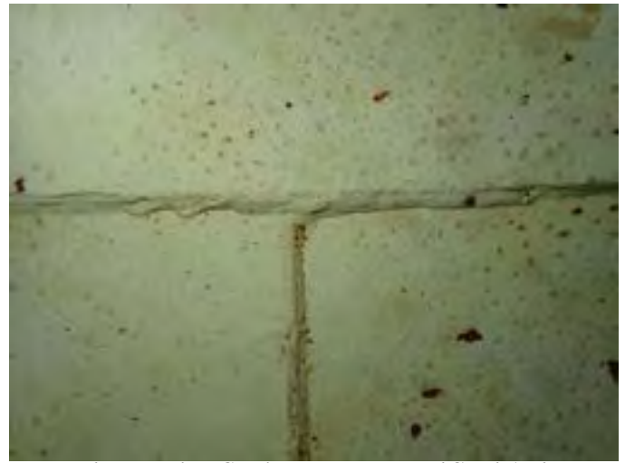
46 Floor Having Coating Loss, Exposed Steel And Corrosion
