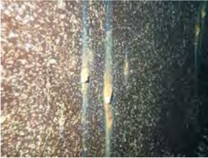
57 Interior Wall Having Coating Fatigue, Exposed Steel And Corrosion
