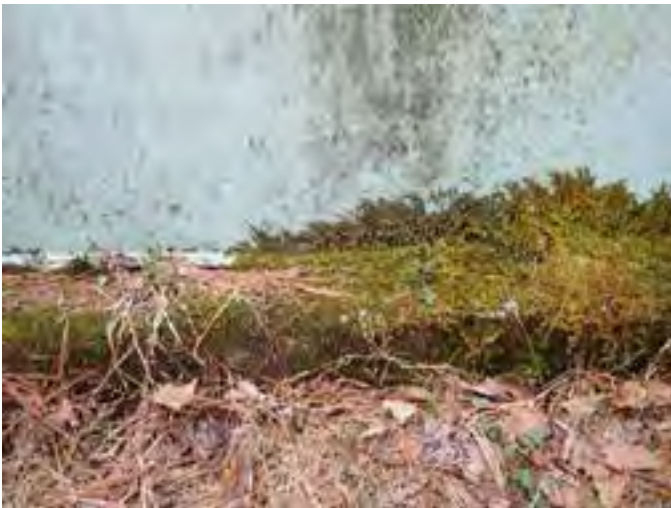
15 Exposed Foundation Surface Found Covered With Moss And Vegetation
