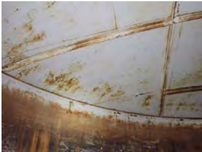
81 Overhead Having Coating Loss, Exposed Steel And Corrosion
