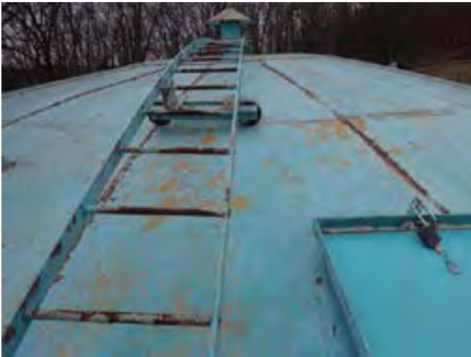
19 Ladder Extending From The Vent Having Exposed Steel And Corrosion
