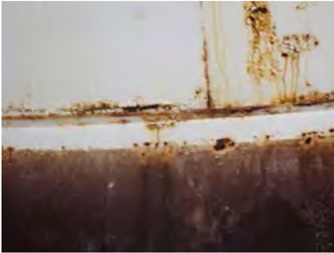
61 Interior Wall Having Exposed Steel And Corrosion
