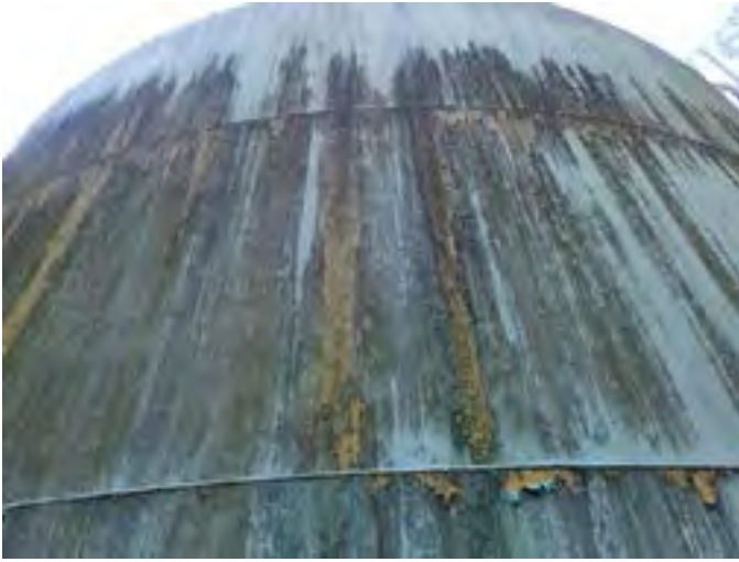
7 Exterior Wall Having Coating Loss, Exposed Primary Coating And Accumulated Mildew
