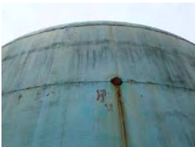
5 Steel Patch Welded Over A Weld Found Without Leakage
