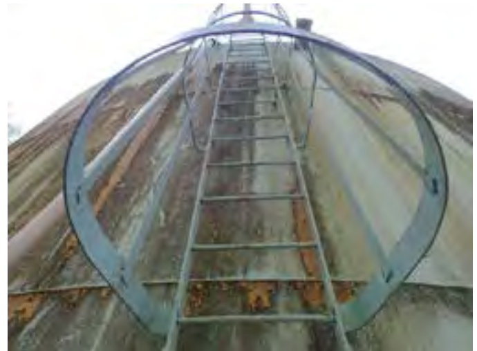
22 Ladder And Safety Cage Having Exposed Steel And Corrosion
