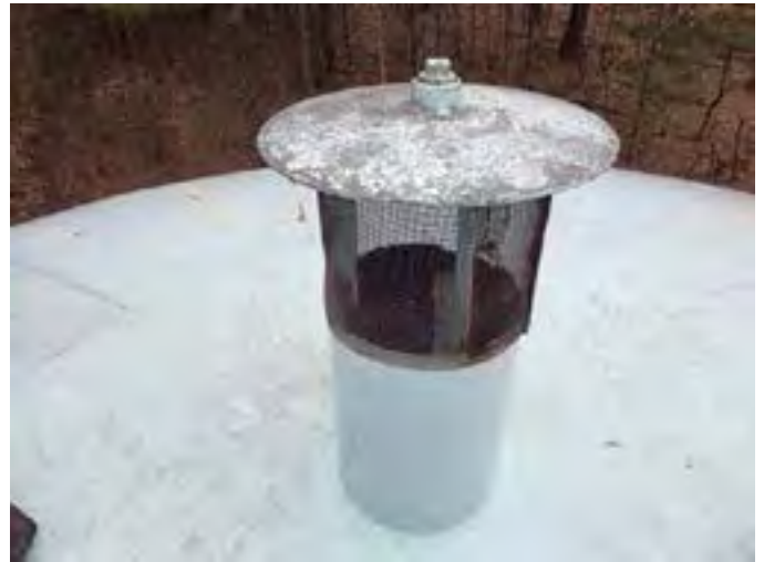
34 Vent Assembly Having Exposed Steel And Corrosion
