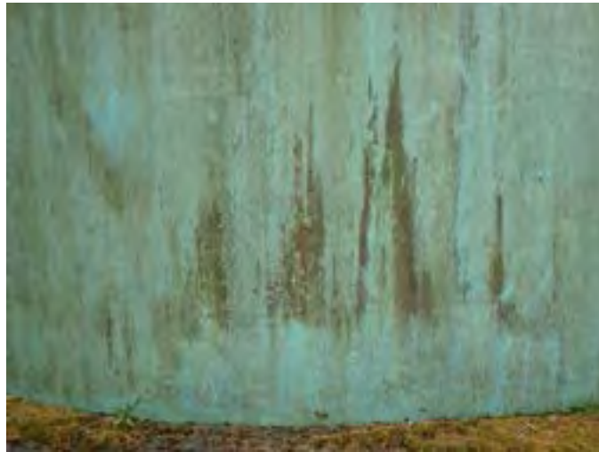
9 Exterior Wall Having Coating Loss, Exposed Primary Coating, Exposed Steel, Corrosion And Accumulated Mildew
