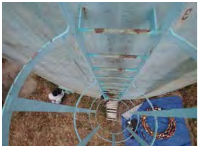
18 Ladder And Safety Cage Having Exposed Primary Coating, Exposed Steel And Corrosion
