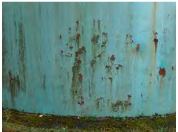
4 Exterior Wall Having Coating Loss, Exposed Primary Coating, Exposed Steel, Corrosion And Accumulated Mildew
