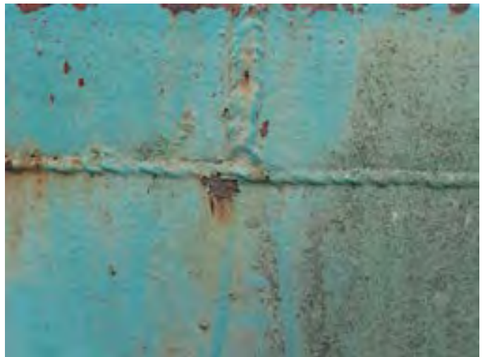
6 Exterior Wall Having Coating Loss, Exposed Primary Coating, Exposed Steel, Corrosion And Accumulated Mildew
