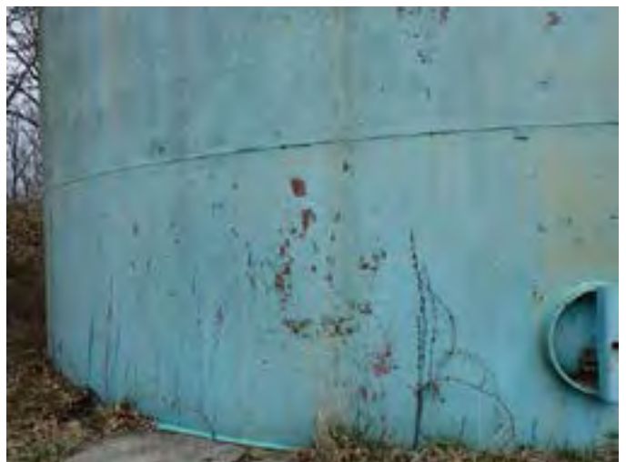
6 Exterior Wall Having Coating Fatigue, Exposed Primary Coating, Exposed Steel And Corrosion
