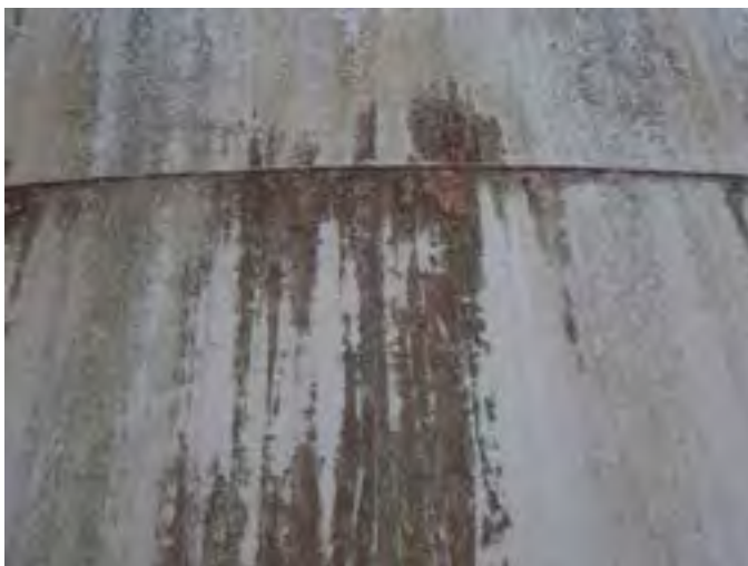
5 Exterior Wall Having Coating Loss, Exposed Primary Coating And Accumulated Mildew
