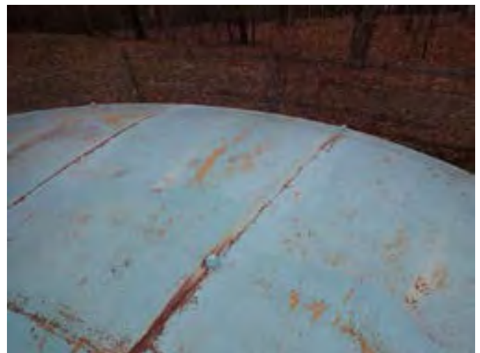
24 Roof Having Exposed Primary Coating, Exposed Steel And Corrosion
