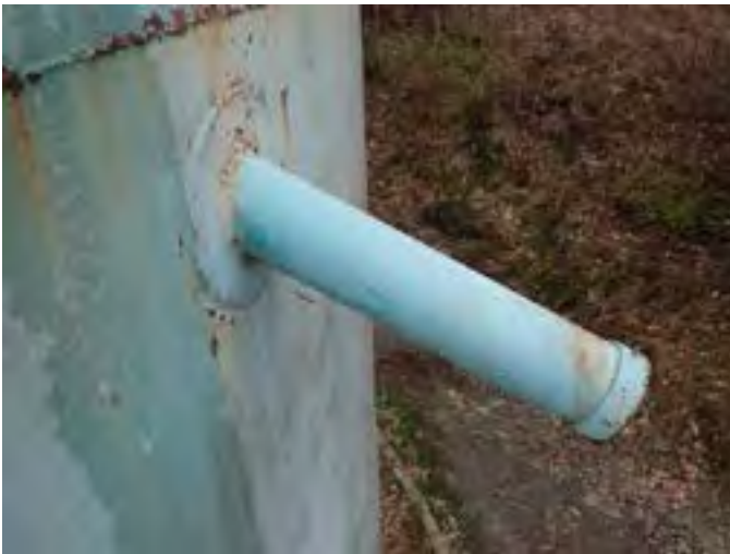
21 Overflow Pipe Having Exposed Primary Coating, Exposed Steel And Corrosion
