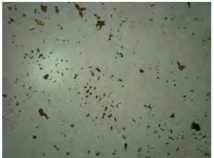
40 Floor Having Coating Loss, Exposed Steel And Corrosion
