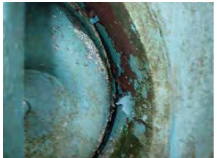
18 Manway Having Exposed Primary Coating
