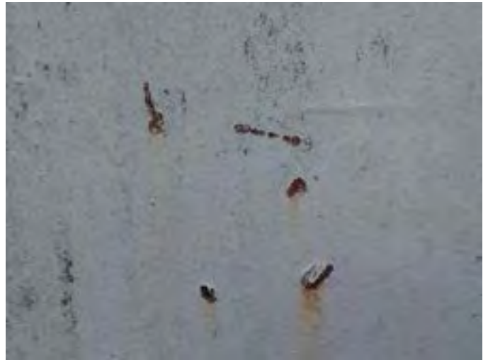
14 Exterior Wall Having Coating Loss, Exposed Steel And Corrosion
