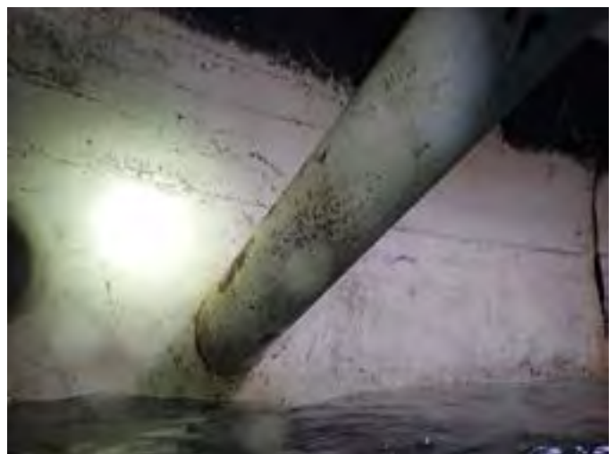
72 Overflow Pipe Having Exposed Steel And Corrosion
