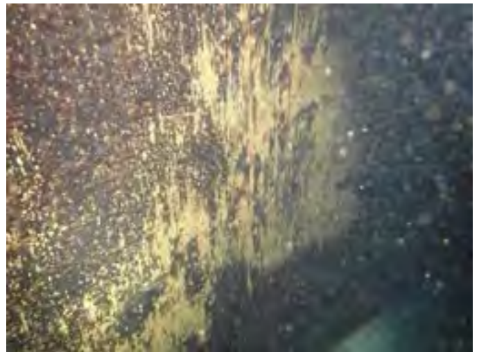
58 Interior Wall Having Coating Loss, Exposed Steel And Corrosion
