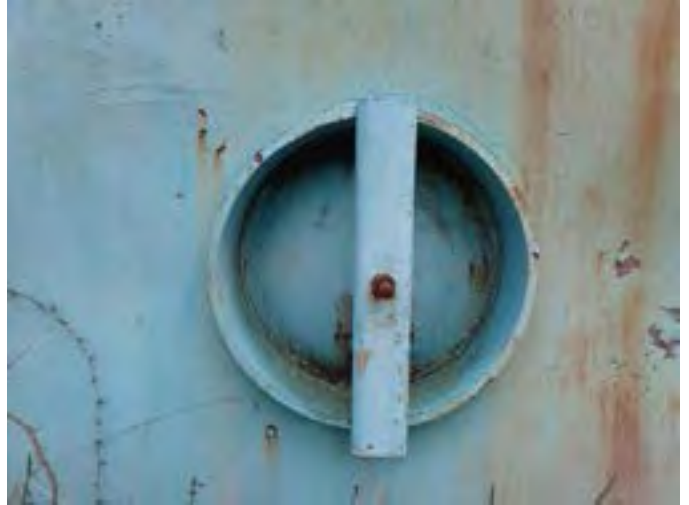
16 Manway Having Exposed Primary Coating, Exposed Steel And Corrosion
