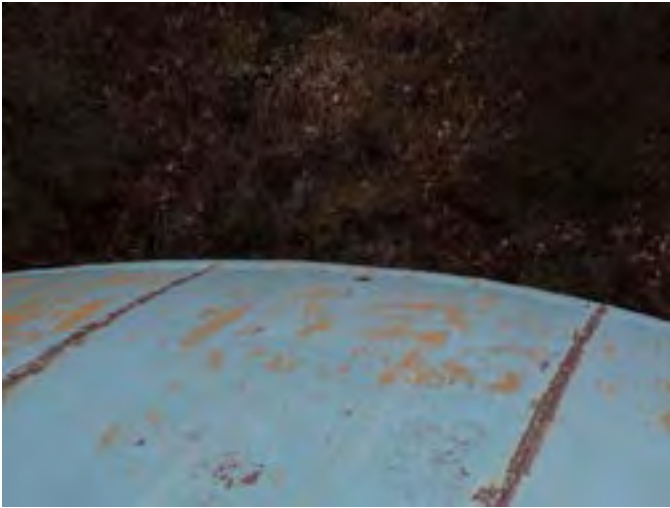
31 Open Rigging Hole Penetration Within The Roof
