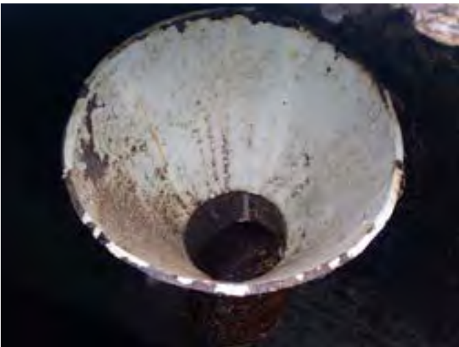
89 Unobstructed Overflow Pipe
