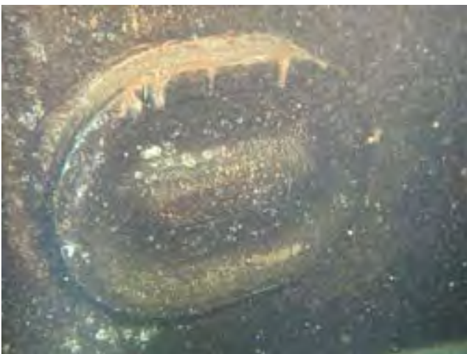
53 Manway Having Coating Loss, Exposed Steel And Corrosion
