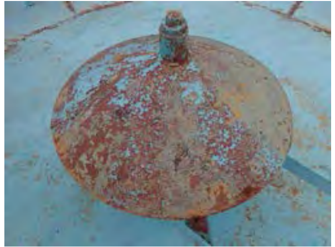
32 Vent Assembly Having Exposed Primary Coating, Exposed Steel And Corrosion
