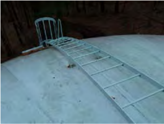
25 Vent Access Ladder Having Exposed Steel And Corrosion
