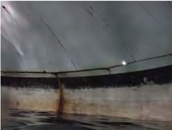
69 Overhead Having Exposed Steel, Corrosion And An Open Rigging Hole Penetration
