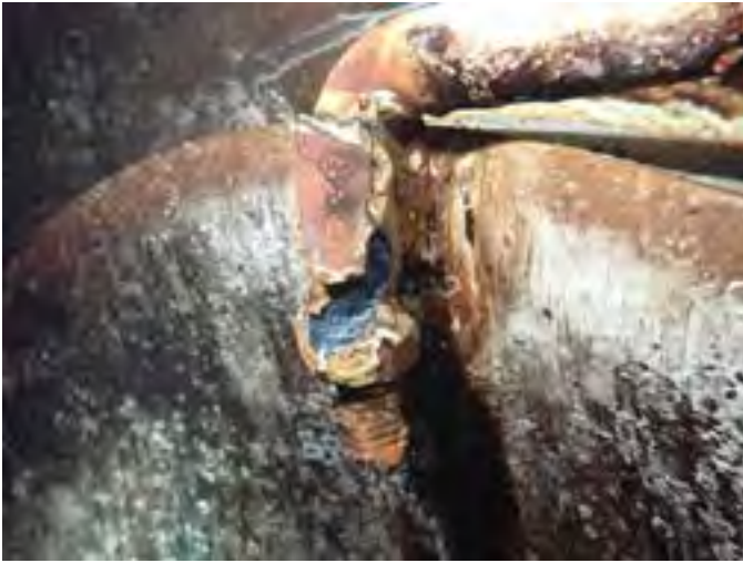
49 Manway Davit Hinge Assembly Exposed Steel, Corrosion And Deterioration Of The Steel
