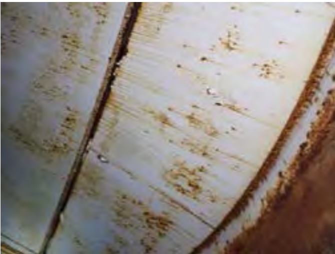
87 Overhead Having Coating Loss, Exposed Steel And Corrosion
