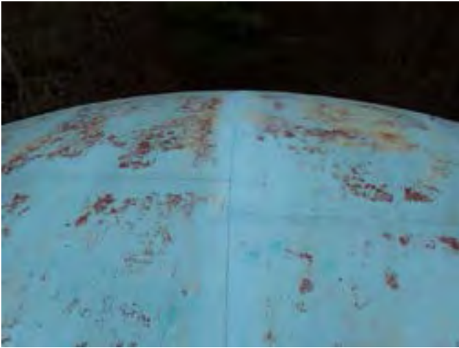
25 Roof Having Coating Fatigue, Exposed Primary Coating, Exposed Steel And Corrosion
