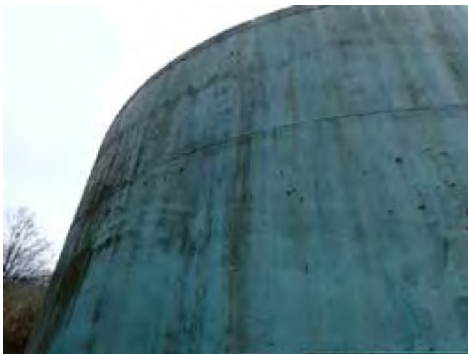
11 Exterior Wall Having Coating Fatigue, Exposed Primary Coating, Exposed Steel And Corrosion
