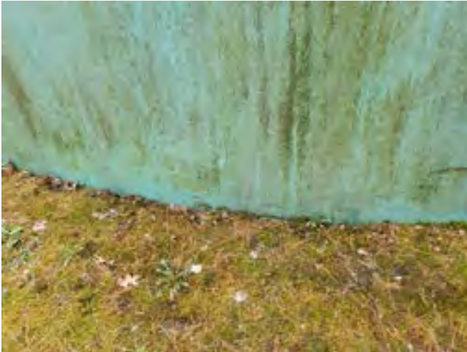
15 Foundation Found Below Grade And Covered With Moss And Vegetation
