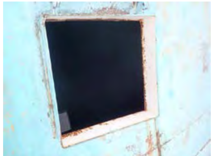
36 Interior Of The Hatch Trunk Having Exposed Steel And Corrosion
