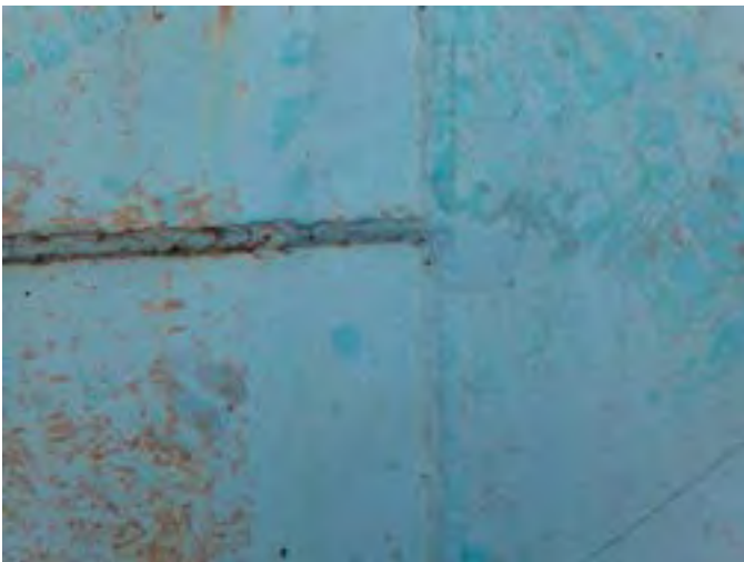
29 Roof Having Coating Fatigue, Exposed Primary Coating, Exposed Steel And Corrosion
