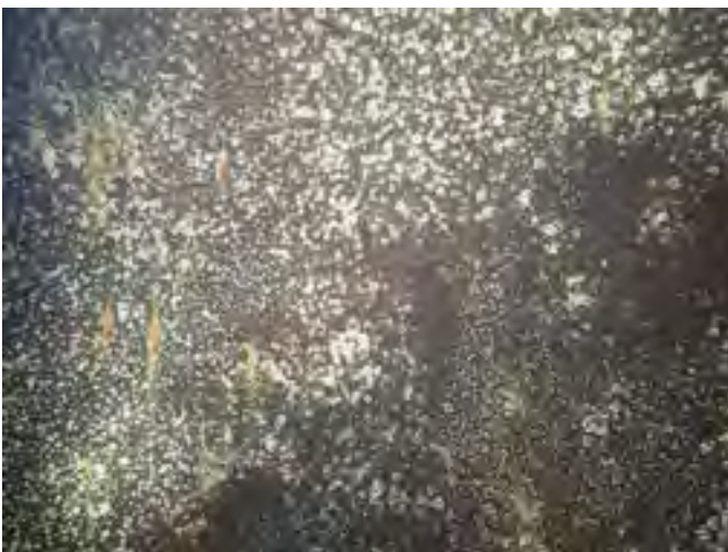
53 Interior Wall Having Exposed Steel And Corrosion
