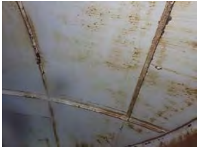
82 Overhead Having Coating Loss, Exposed Steel And Corrosion
