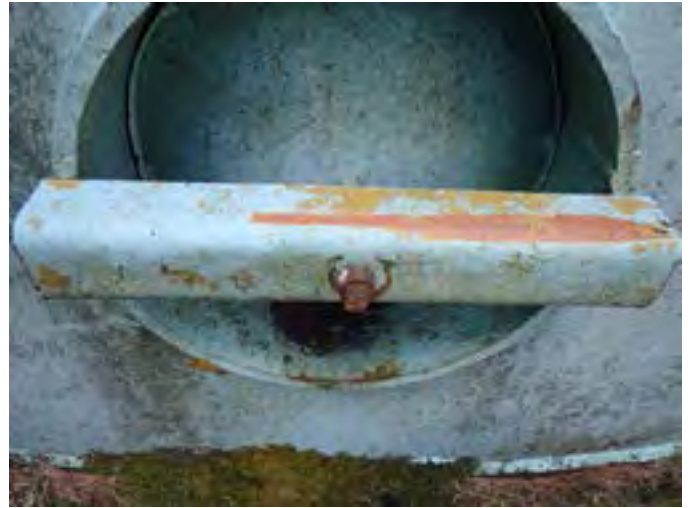
20 Manway Having Exposed Primary Coating
