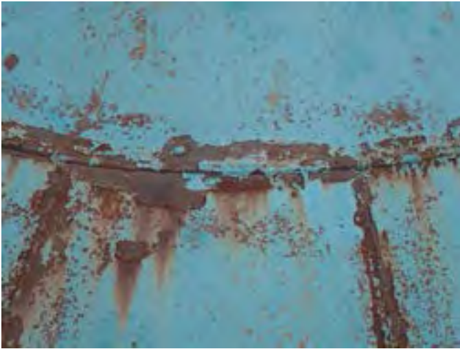
25 Roof Having Exposed Primary Coating, Exposed Steel And Corrosion
