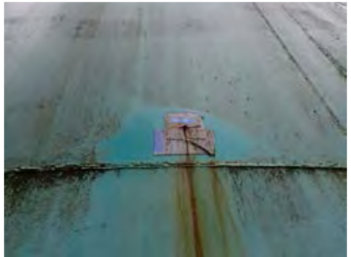
2 Wood Dowel And Patch Temporarily Sealing A Penetration In The Second Wall Panel On The Southernmost Side Of The Tank
