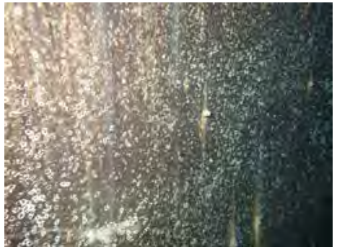
54 Interior Wall Having Coating Fatigue, Exposed Steel And Corrosion
