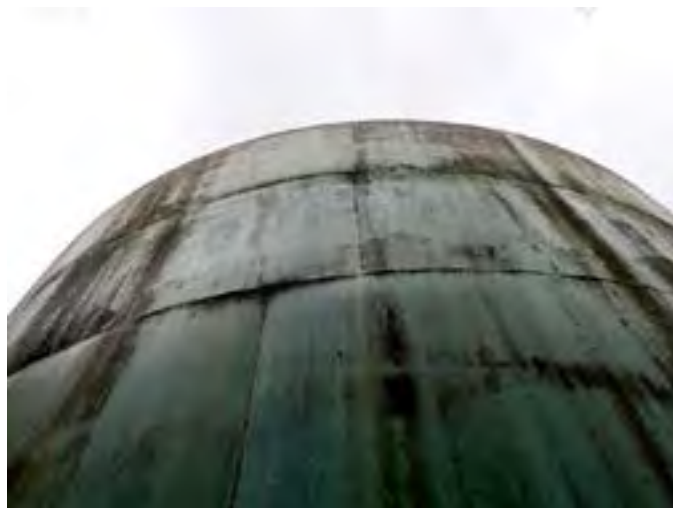
11 Exterior Wall Having Coating Loss, Exposed Steel, Corrosion And Accumulated Mildew
