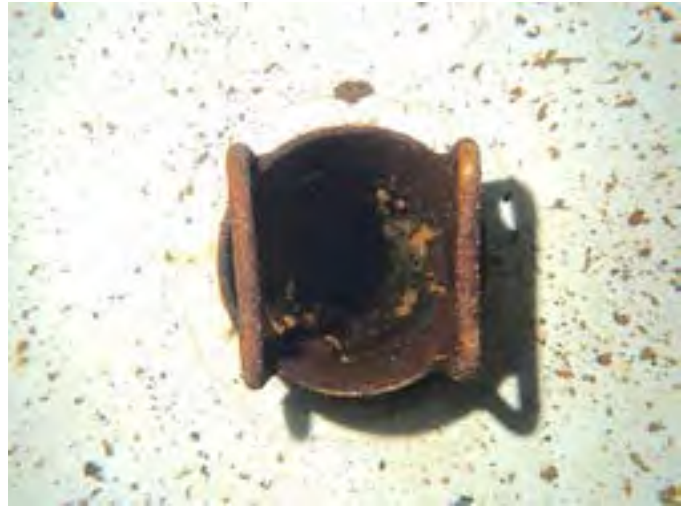
50 Interior Of The Pipe Within The Floor Having Corrosion
