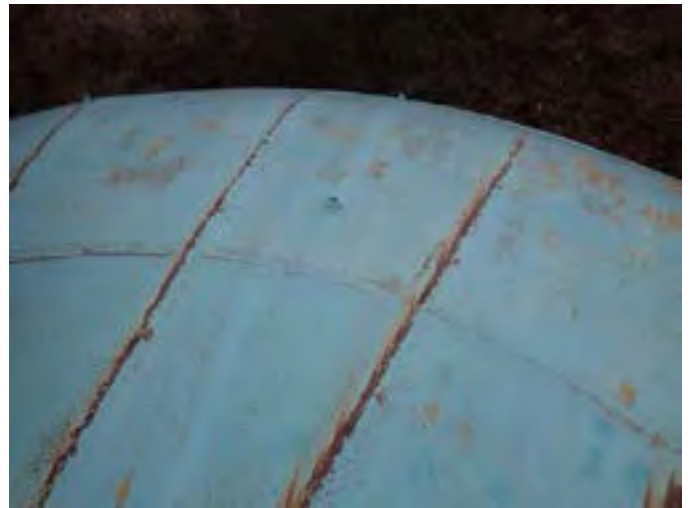
28 Roof Having Exposed Primary Coating, Exposed Steel And Corrosion
