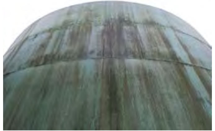
14 Exterior Wall Having Coating Loss, Exposed Steel, Corrosion And Accumulated Mildew
