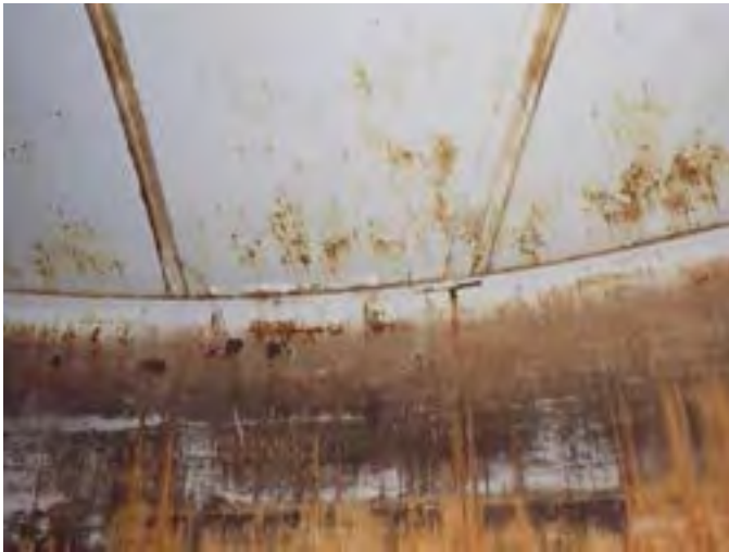
75 Interior Wall Having Coating Loss, Exposed Steel And Corrosion
