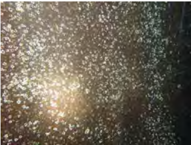
53 Interior Wall Having Coating Fatigue, Exposed Steel And Corrosion
