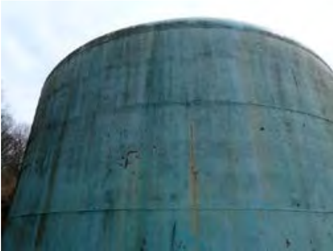
15 Tank Exterior Having Accumulated Mildew
