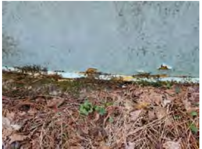
16 Exposed Foundation Surface Found Covered With Moss And Vegetation
