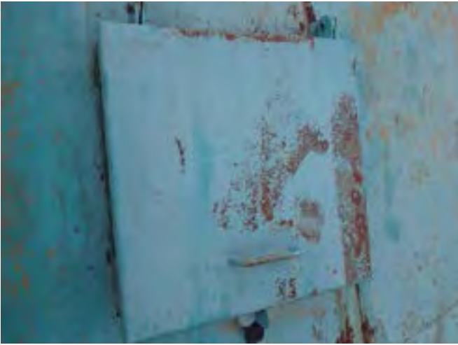
37 Exterior Of The Hatch Cover Having Exposed Primary Coating, Exposed Steel And Corrosion
