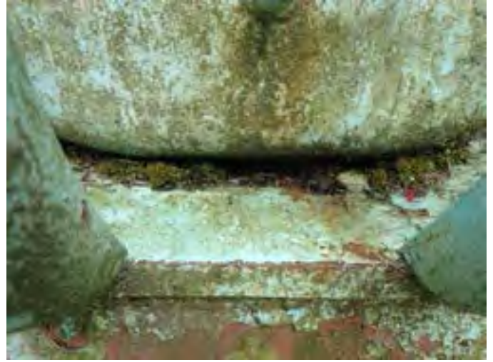
20 Manway Having Mild Leakage At Its Base
