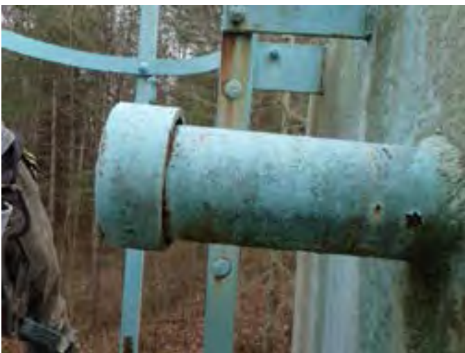
23 Overflow Pipe Having Coating Loss, Exposed Steel And Corrosion
