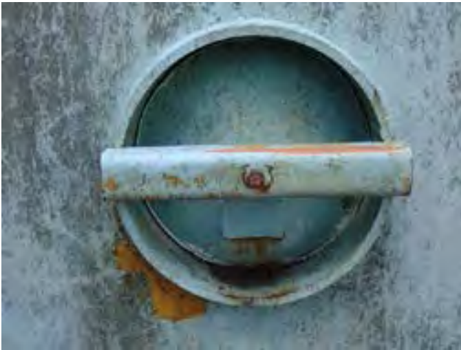
19 Manway Having Coating Loss
