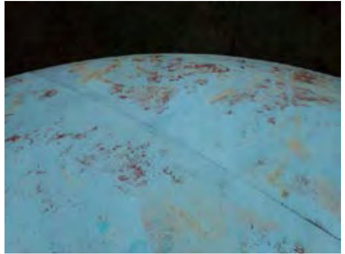
26 Roof Having Coating Fatigue, Exposed Primary Coating, Exposed Steel And Corrosion
