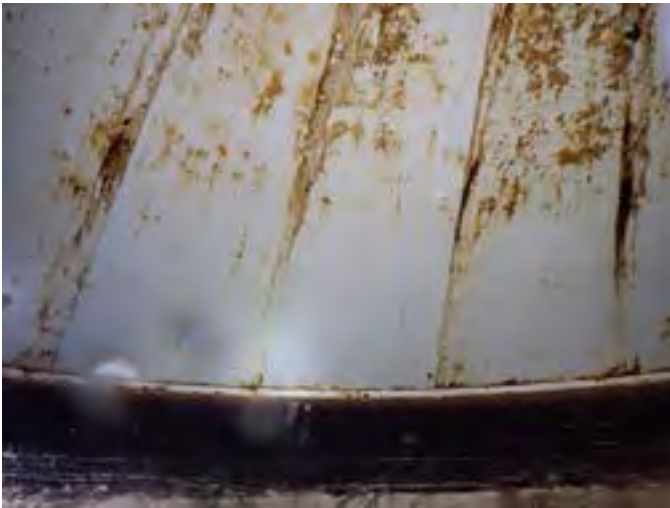
69 Overhead Having Coating Loss, Exposed Steel And Corrosion
