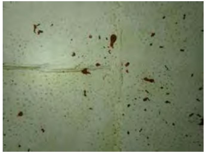
44 Floor Having Coating Loss, Exposed Steel And Corrosion
