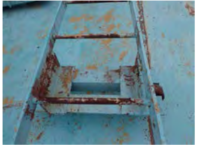
20 Ladder Extending From The Vent Having Exposed Steel And Corrosion
