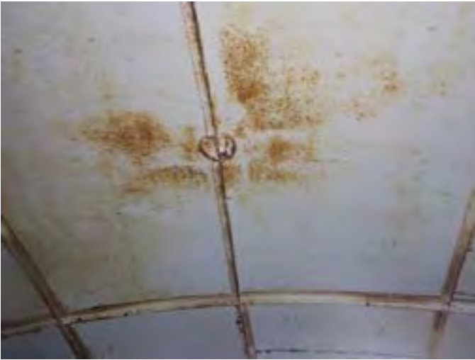
85 Overhead Having Coating Loss, Exposed Steel And Corrosion
