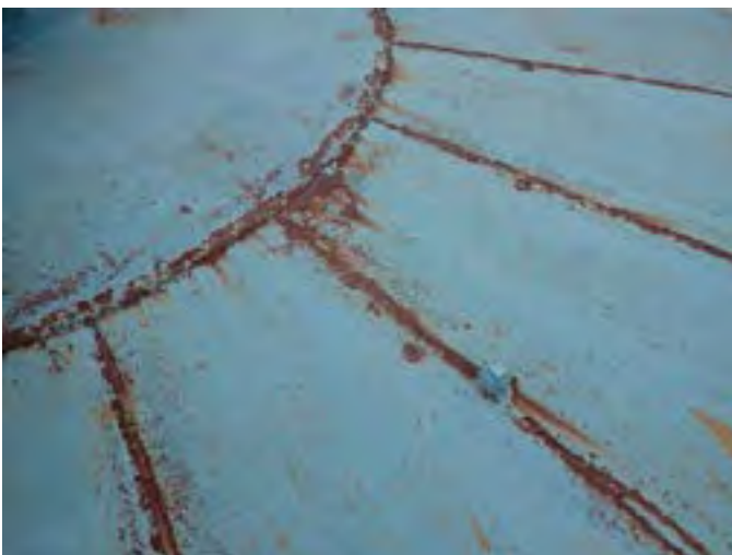
29 Rigging Hole Penetration Sealed With A Threaded Plug
