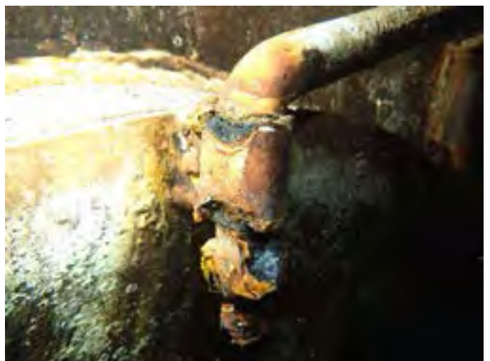
48 Manway Davit Hinge Assembly Exposed Steel, Corrosion And Deterioration Of The Steel
