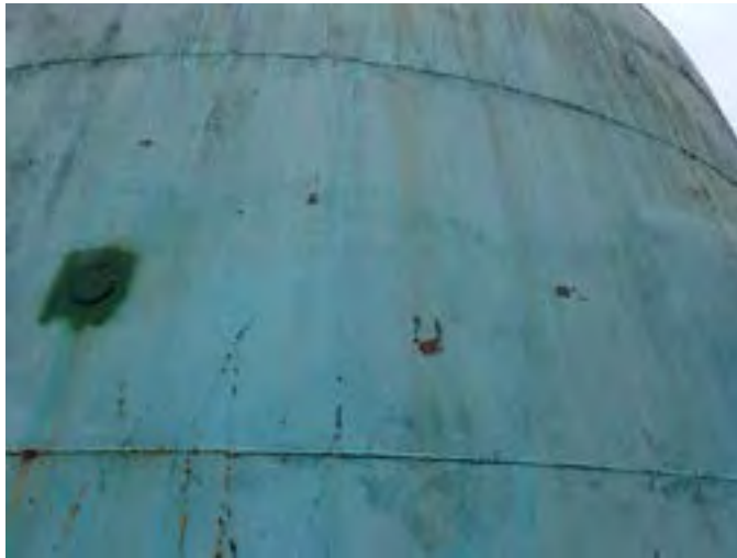
9 Exterior Wall Having Coating Fatigue, Exposed Primary Coating, Exposed Steel And Corrosion
