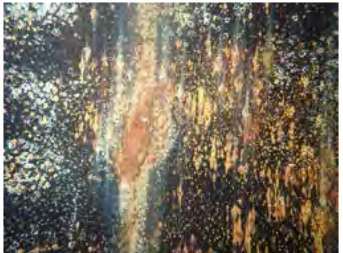
58 Interior Wall Having Exposed Steel And Corrosion
