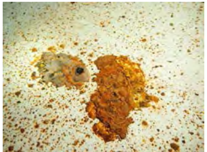
42 Floor Having Coating Loss, Exposed Steel And Corrosion
