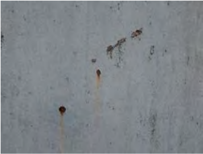
13 Exterior Wall Having Coating Loss, Exposed Steel And Corrosion
