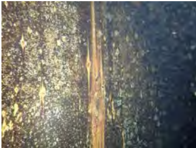
63 Interior Wall Having Coating Loss, Exposed Steel And Corrosion
