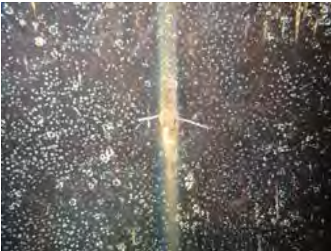
57 Interior Wall Having Exposed Steel And Corrosion
