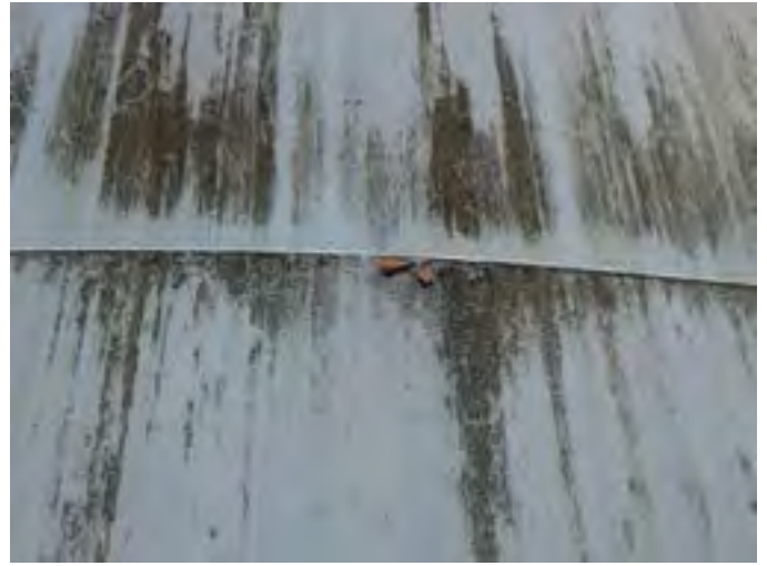
8 Exterior Wall Having Coating Loss, Exposed Primary Coating And Accumulated Mildew
