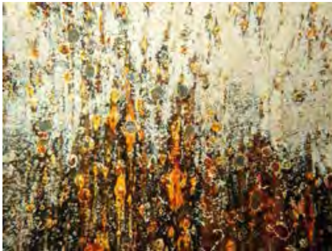
63 Third Row Of Wall Panels Above The Tank Floor Having Pitting Of The Steel
