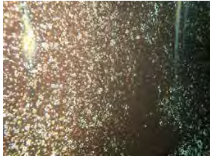
58 Interior Wall Having Coating Fatigue, Exposed Steel And Corrosion
