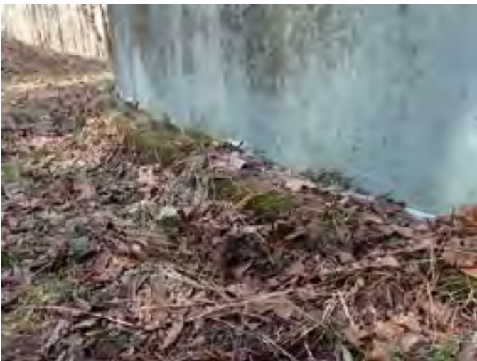
17 Exposed Foundation Surface Found Covered With Moss And Vegetation
