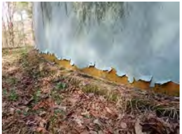
18 Exposed Foundation Surface Found Covered With Moss And Vegetation
