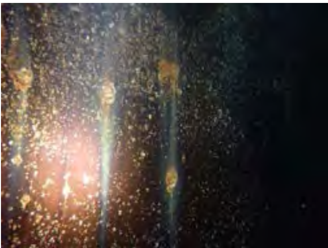
59 Interior Wall Having Coating Fatigue, Exposed Steel And Corrosion
