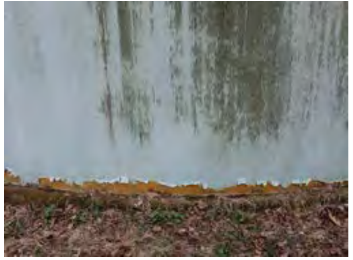
2 Exterior Wall Having Coating Loss, Exposed Primary Coating And Accumulated Mildew
