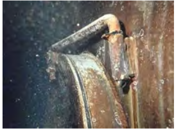
50 Manway Davit Hinge Assembly Exposed Steel, Corrosion And Deterioration Of The Steel
