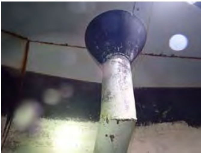
75 Unobstructed Overflow Pipe
