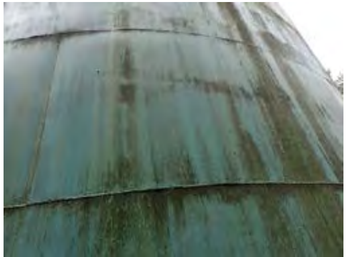
10 Exterior Wall Having Coating Loss, Exposed Steel, Corrosion And Accumulated Mildew
