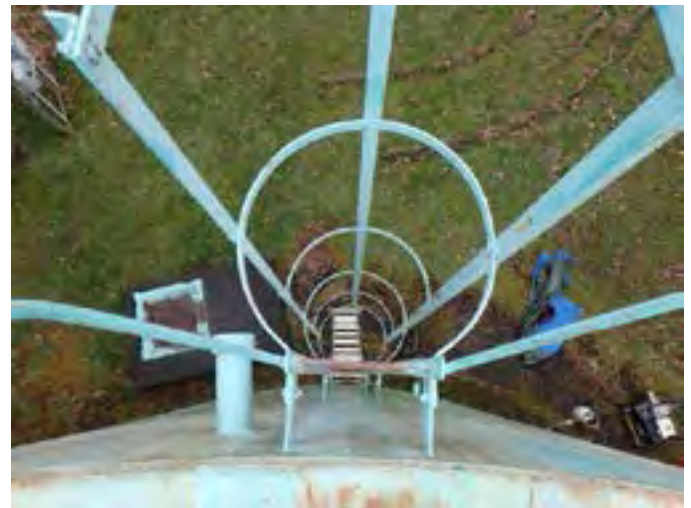
22 Ladder And Safety Cage Having Coating Loss, Exposed Steel And Corrosion
