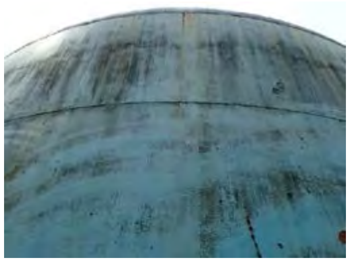
14 Exterior Wall Having Coating Fatigue, Exposed Primary Coating, Exposed Steel And Corrosion
